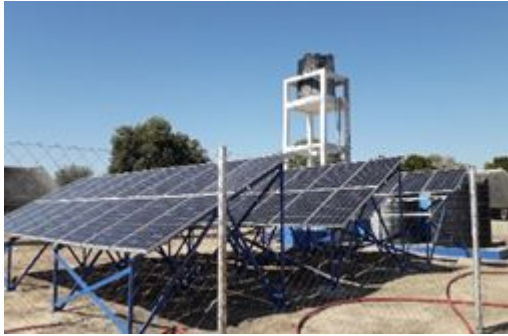
Artesian well in Mahatlane ( Chicualacuala region) - water for 559 people
